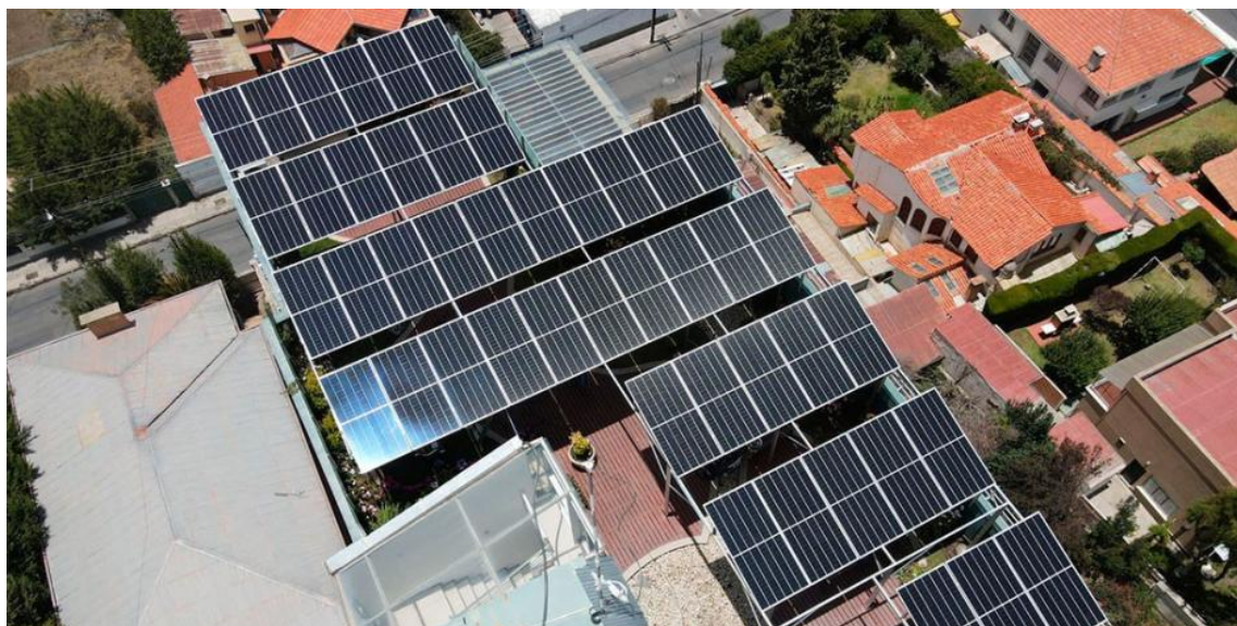
Solar panels at the national office of CRECER IFD
